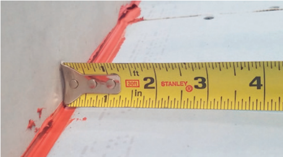
Fig. 30: Inadequate width of the sealant/gap
