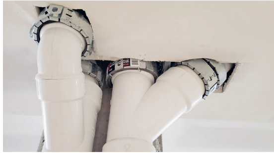
Fig. 15: Multiple cable collars Hilti CP-643 N used for sealing a large opening, leaving gaps in the installation
