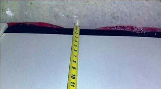
Fig. 31: Head of wall joint – width exceeded listed system
