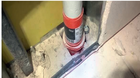
Fig. 17: Hilti CP 680 sleeve not cast into concrete
