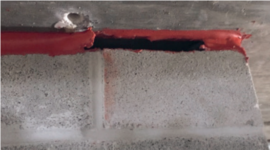
Fig. 29: Gap in application
