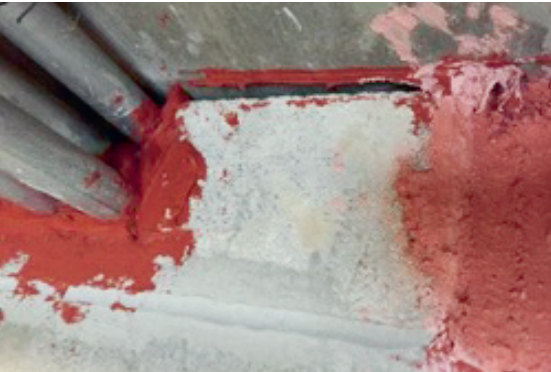
Fig. 35: Cracked sealant coating
