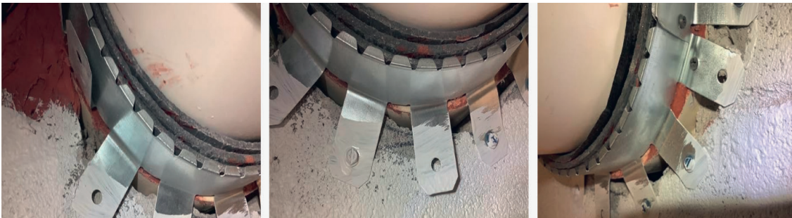
Fig. 18: Gaps in opening exist
