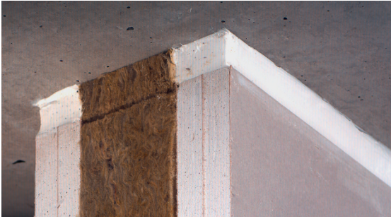
Fig. 22: Flexible firestop sealant (Hilti CP606 - white) applied to both sides of the wall with mineral wool backing material
