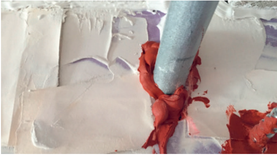
Fig. 14: Sealant not properly tooled leaving gaps in the installation
